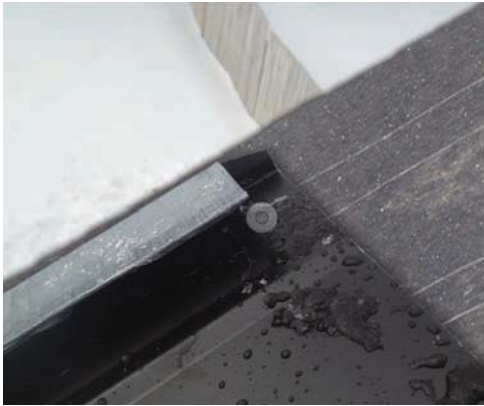
Cut bottom of inner gable so outside weeping channel will protrude past drip edge 1/4".
